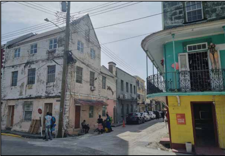
Fig. 2 One of the oldest brick buildings in Bridgetown (17th century), with a poorly thought out roof repair that has made the historic Dutch gable disappear from view (picture by De Waal, February 8, 2024).
